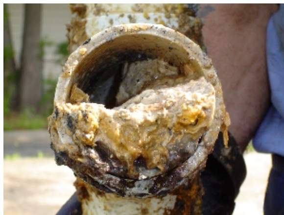
Figure 1: Sanitary sewer line clogged with grease.
